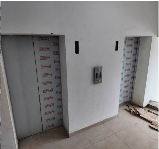
Block B Lift
