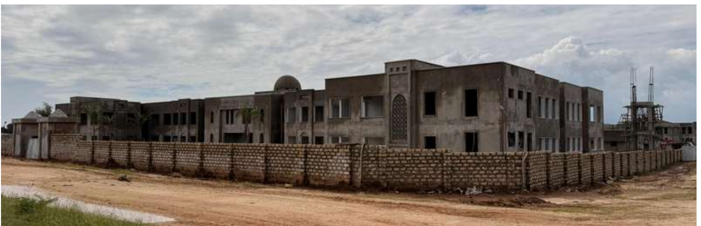
Supporting infrastructure The International School at Vipingo
