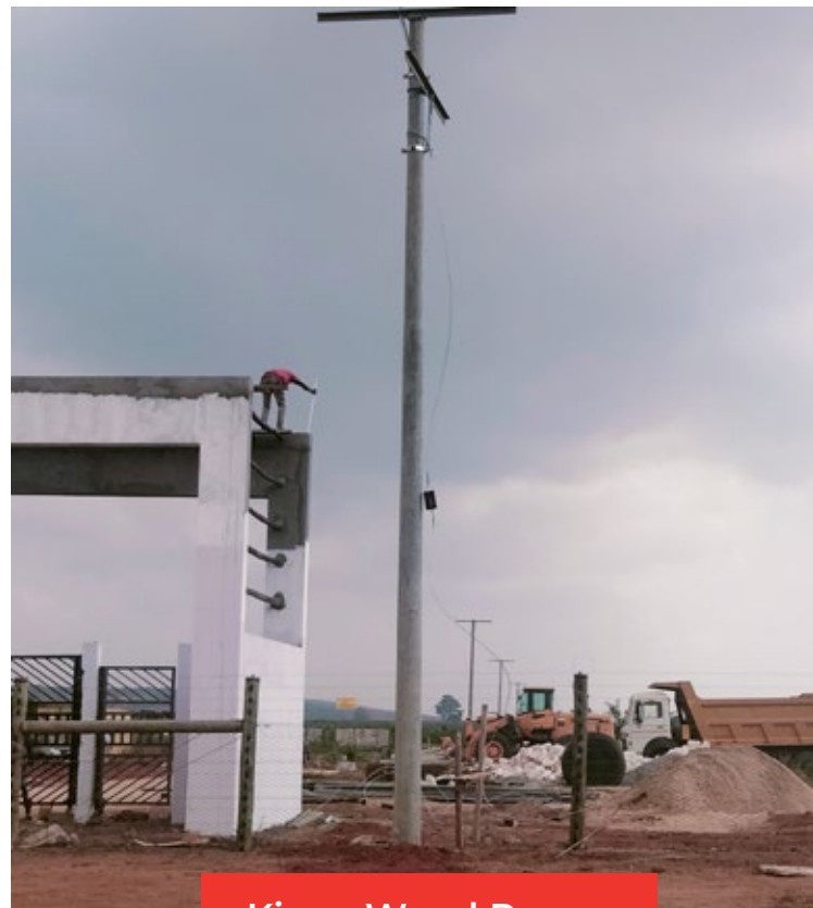
Kings Wood Power connection by KPLC
